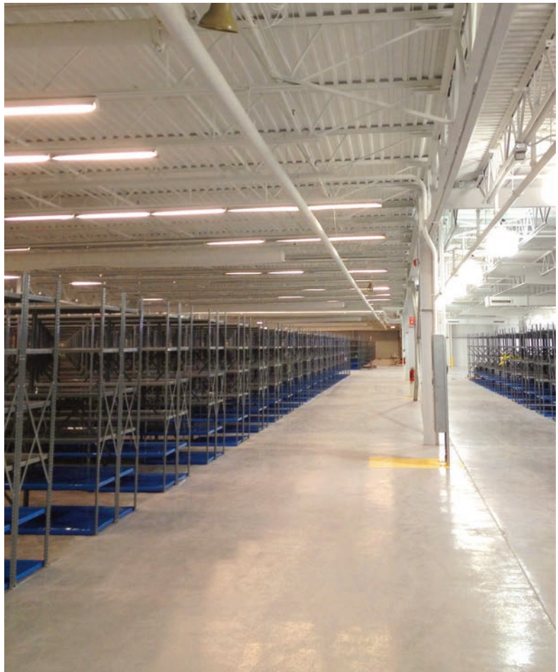
This picture shows the WPSS Deluxe shelving designed to support the conveyor system from the top of the sections prior to the installation of the conveyor system.
